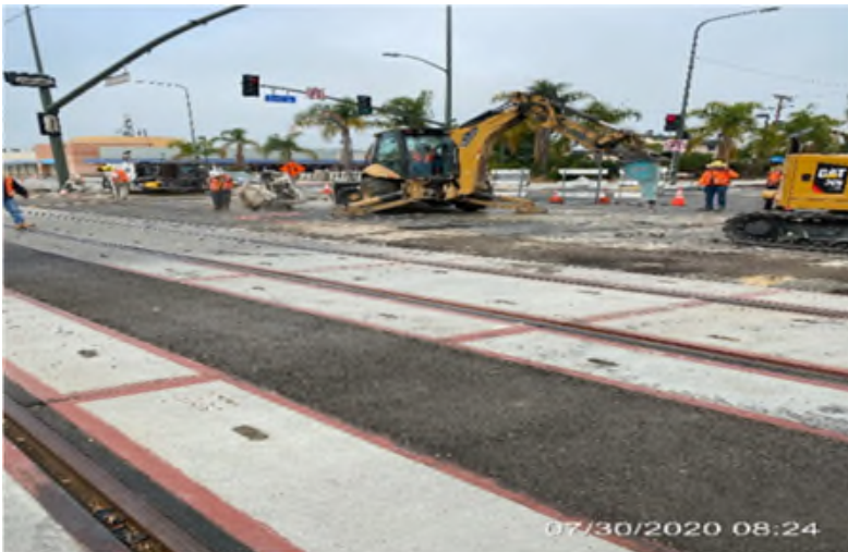
Excavating/removing section of pavement for restoration on southbound Crenshaw Blvd and 54th St.
