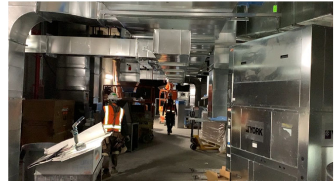
North Mechanical Room Lower Ancillary Level at Grand Av Arts/Bunker Hill Station
