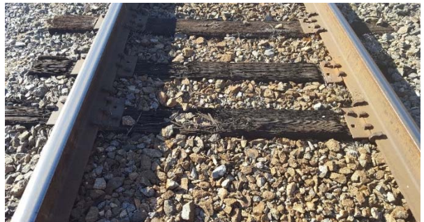
Picture 3: Failed Tie Condition on the Valley Subdivision
