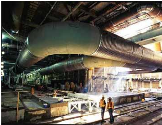
Figure 4-19: Underground Ventilation Ducts
