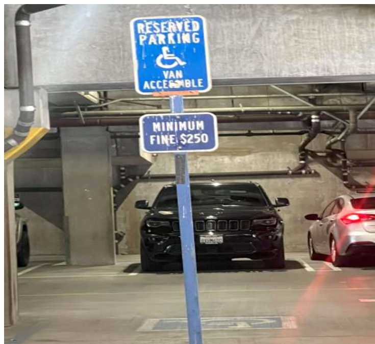
Picture 14 3/11/2026 - Union Station Worn Out Sign/Some Deterioration
