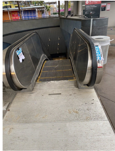
Escalators were shut off at 5 stations for safety reasons
