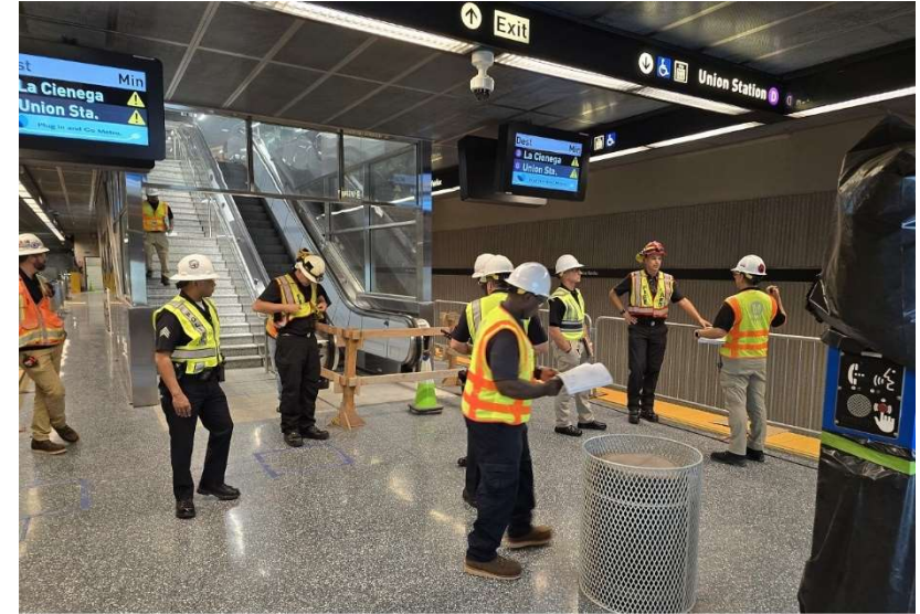
Emergency Drills Prep at Wilshire/Fairfax Station
