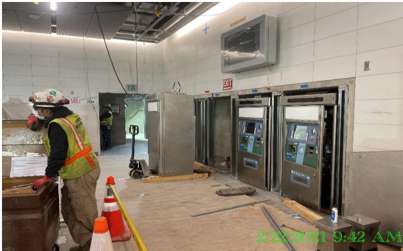
EXPO STATION – Installing and performing electrical work to the ticket vending machines at the Free Area.
