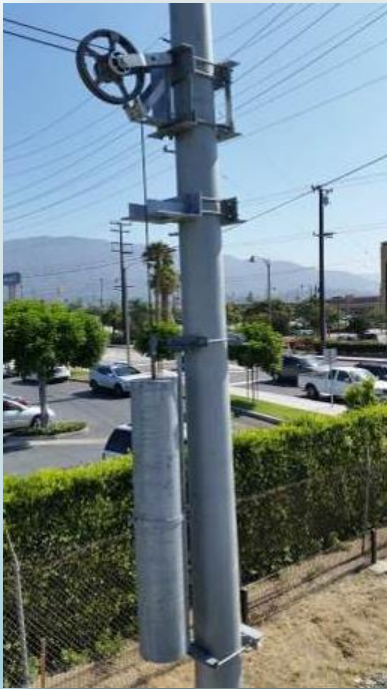
(4) Existing Weight Stack Tensioning System
