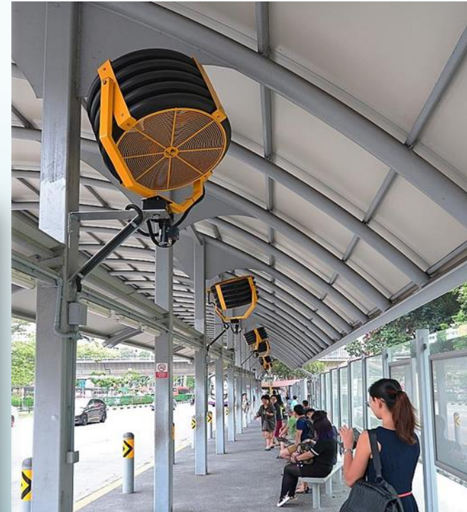
(10) Electric fans at bus stop
