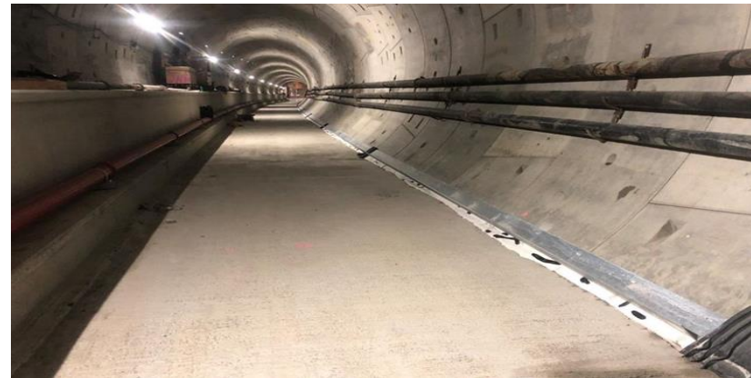
Reach 3 Tunnel (Fairfax to La Cienega) Preparation for North Tunnel Track Layout
