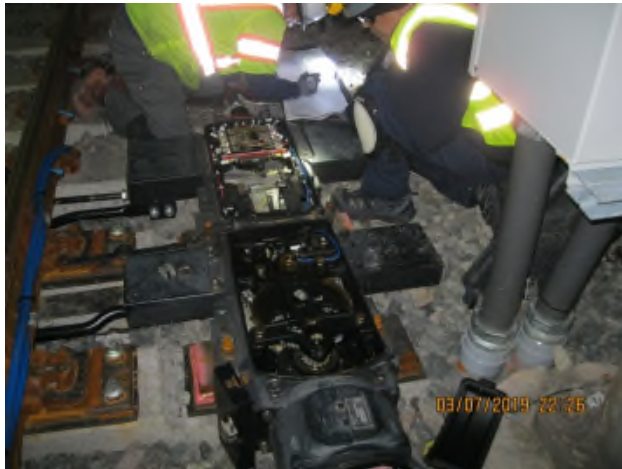
Switch Machine LFAT
