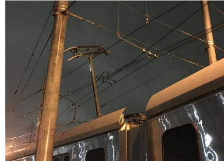
Figure 16: Pantograph entanglement with OCS wires
