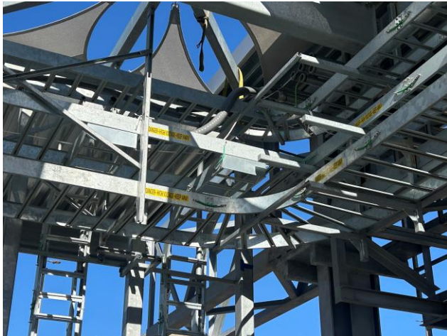
Photo showing Conduit and Shade Sails of the Charging Station
