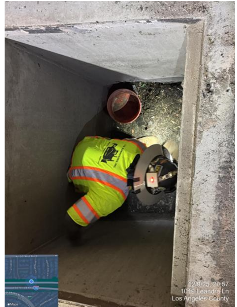
Irrigation pullbox per Punchlist (Arcadia)
