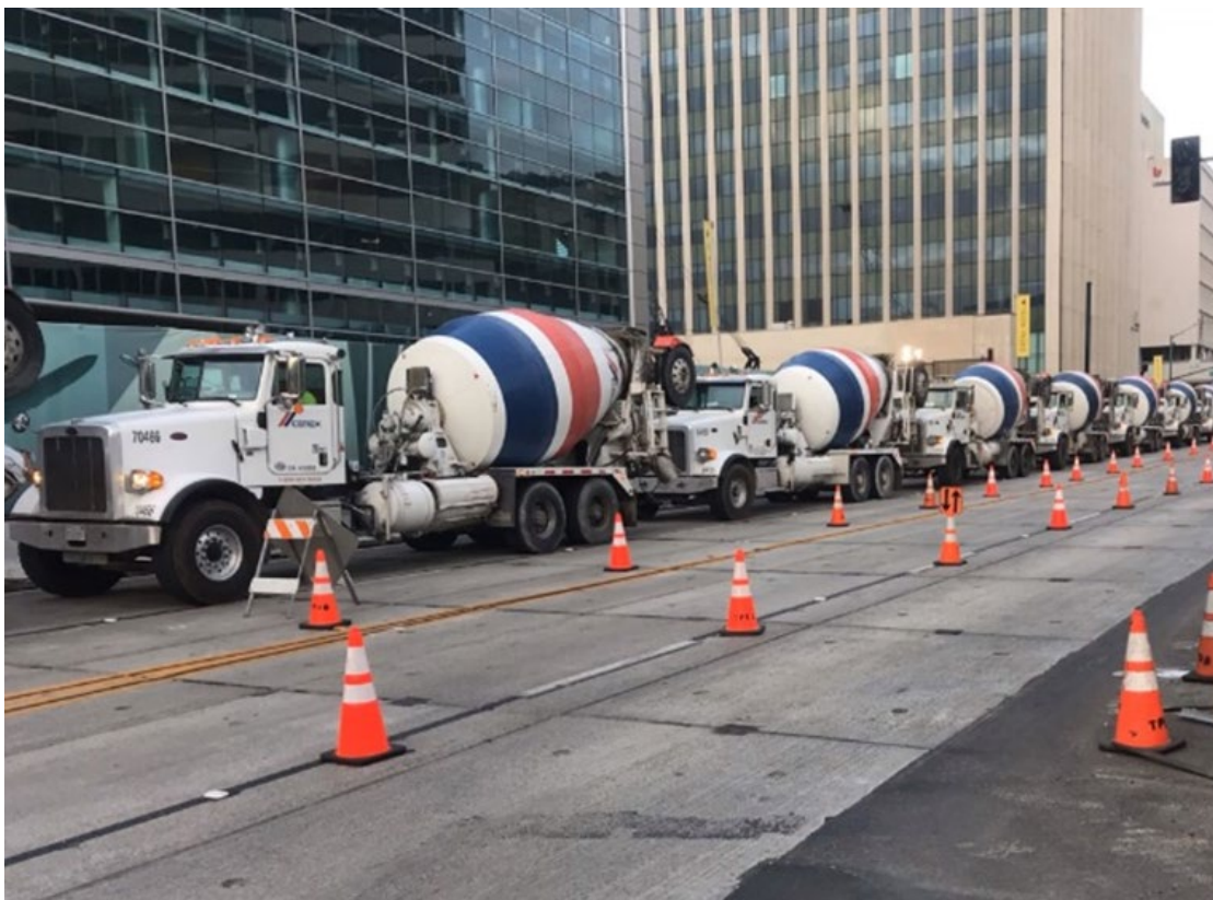
Concrete trucks on Wilshire Blvd awaiting delivery to Rodeo station for concrete slab
