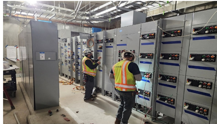
Wilshire/Fairfax Testing Motor Control Center
