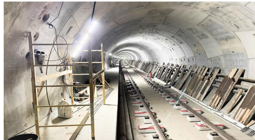
Reach 3 Tunnel (Fairfax to La Cienega) Direct Fixation Blocks and Track Installation
