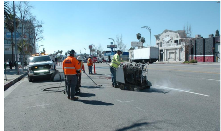
W.A. Rasic crew saw cutting pavement on Van Nuys Blvd. near Hartland St.
