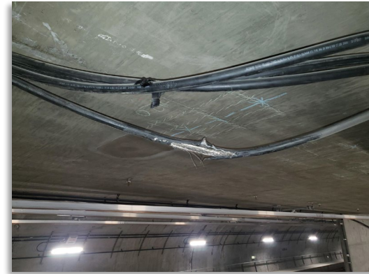
Failed feeder cable securement
