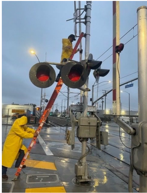
Crews pinned crossing gates in anticipation of high winds
